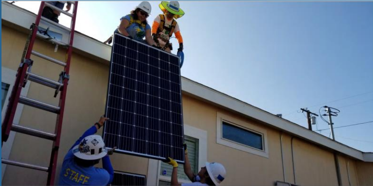
Rooftop solar p.v. panels installed by GRID Alternatives staff and trainees. Photo credit: GRID Alternatives
