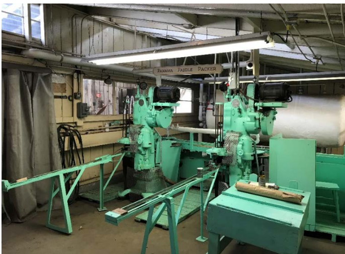
Image 7. The two Panama Paddle Packers machines (Resource No. 22) located on the Canning Room of building resource No.2.
