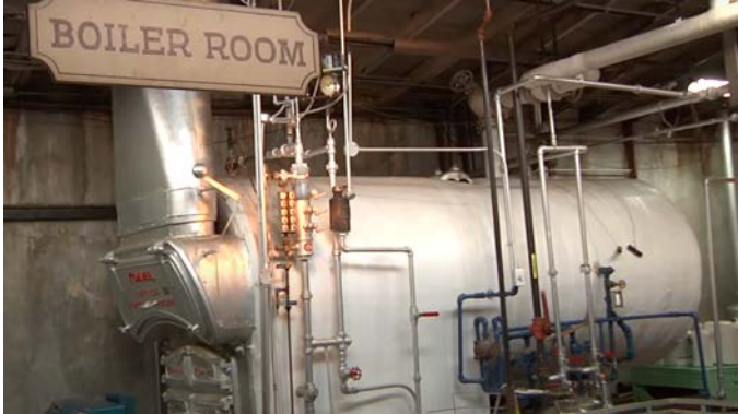
Image 9. View of the Boiler Machine (Resource No. 23) located on the Boiler Room of building resource No. 5.
