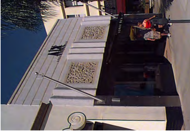
Vertical molding and facade detailing is typical of the Art Deco era.
