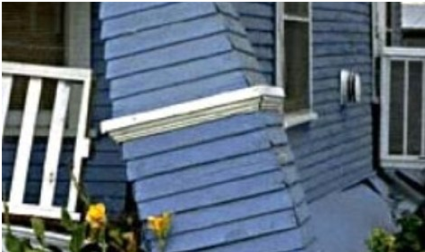
Figure 4-16: Earthquakes can be so strong they knock houses and buildings off their foundation.
