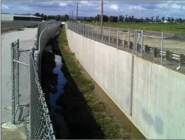
PHOTOGRAPH 1: View of the County Line Channel located to the south of the study area, facing southwest (jurisdictional).
