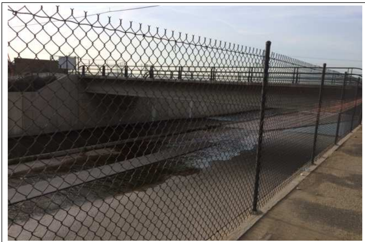
Photograph 3: View of existing Chino Avenue crossing at Cucamonga Creek Flood Control Channel.
