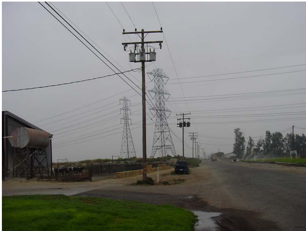
View of pole mounted transformers on the south property boundary along Eucalyptus Avenue.
