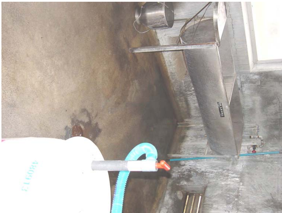
View of the tank room within the milking barn.
