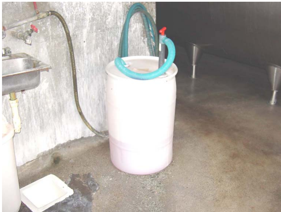
View of 55-gallon plastic drum of acid cleaner within the tank room.
