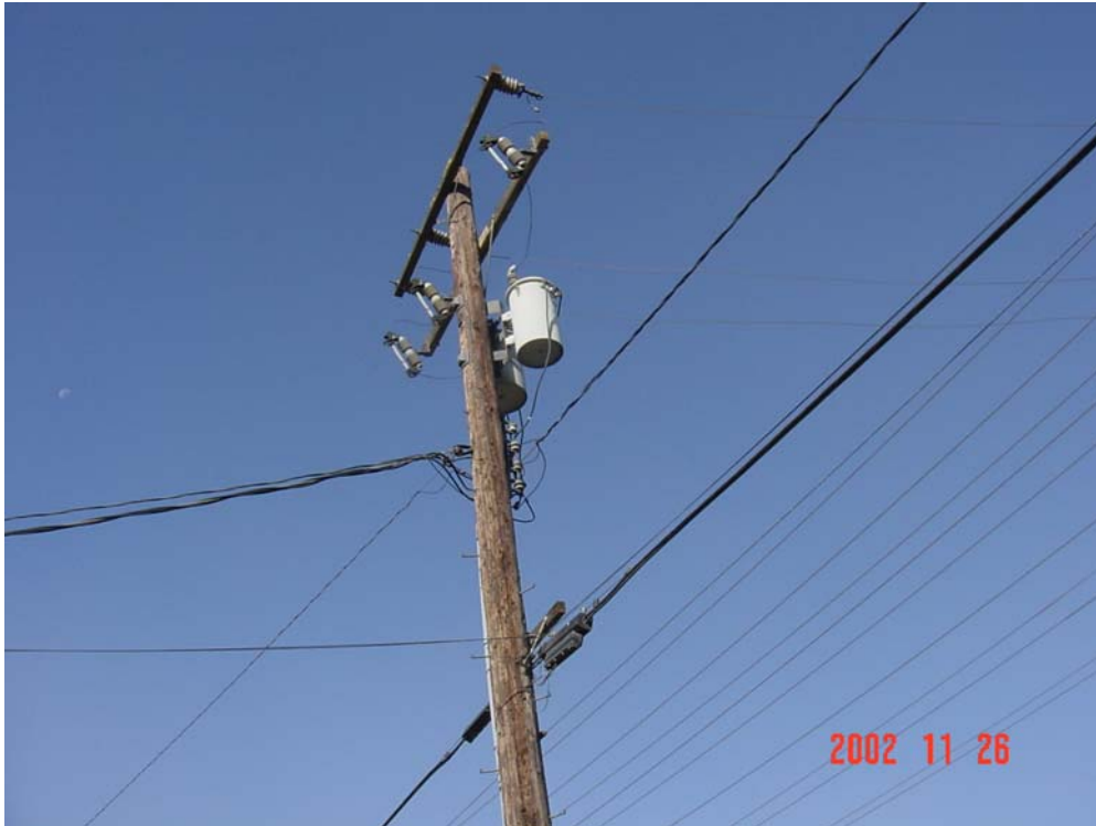
Overview Of Pole Mounted Transformer.
