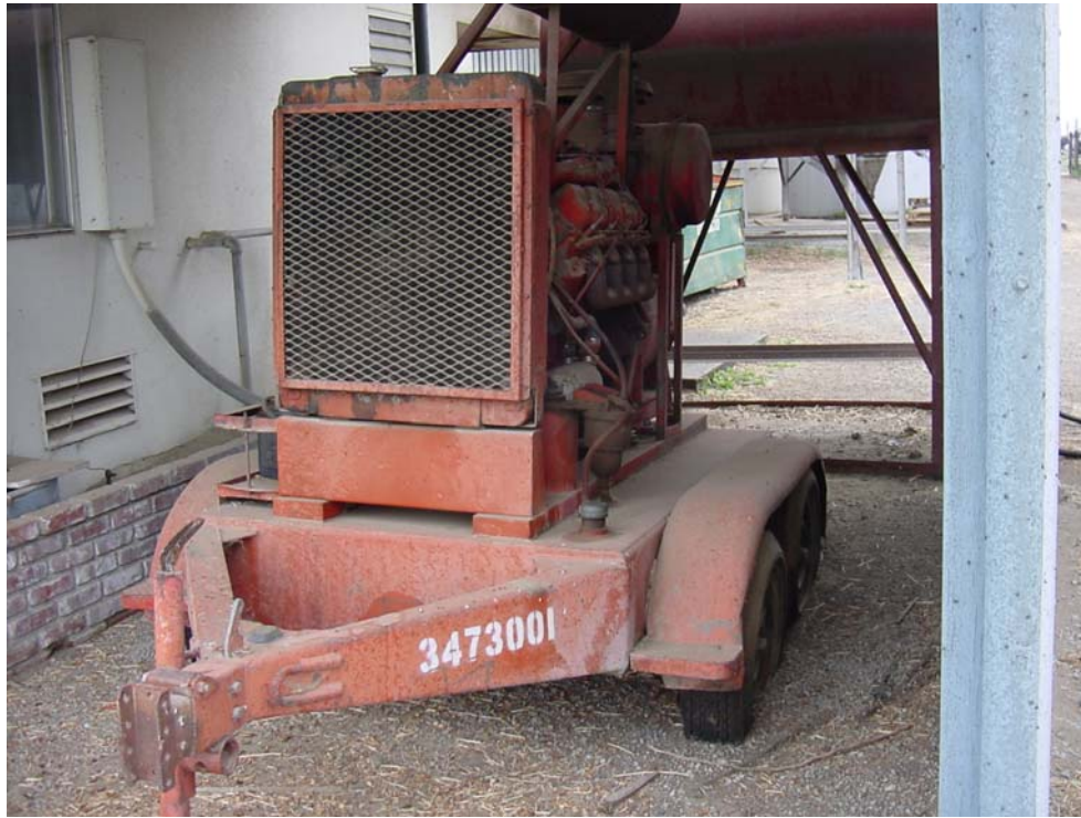
Close-up view of the emergency generator.
