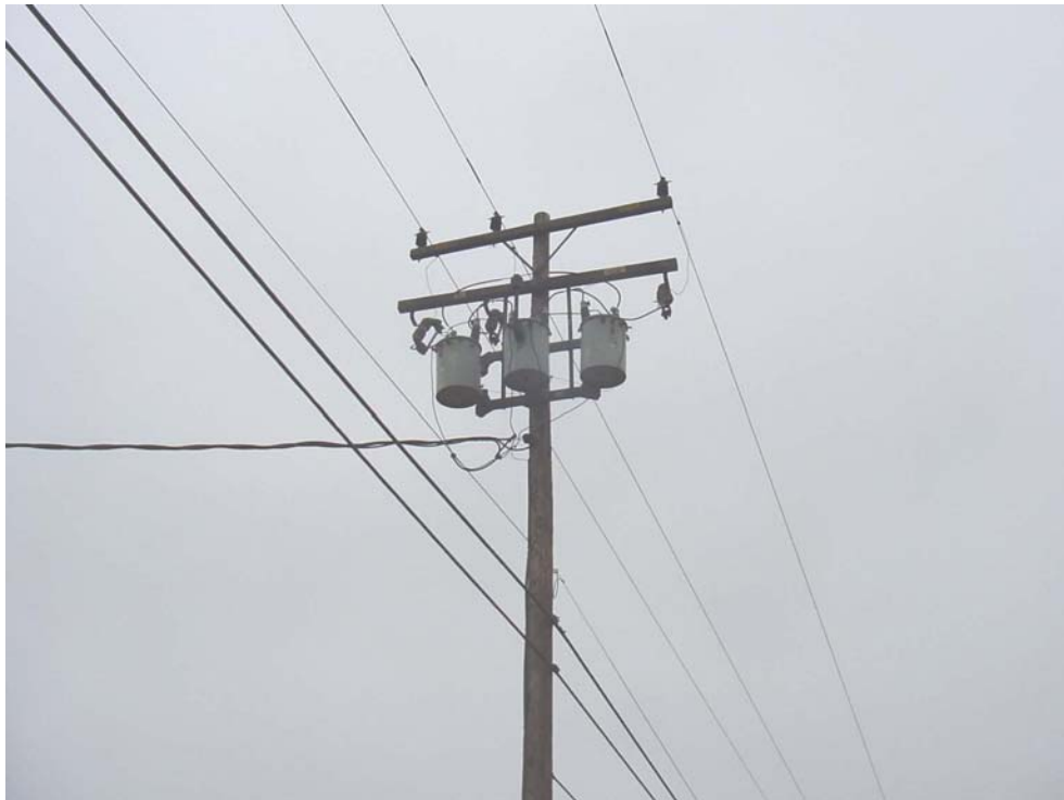
Close-up view of pole mounted transformers.
