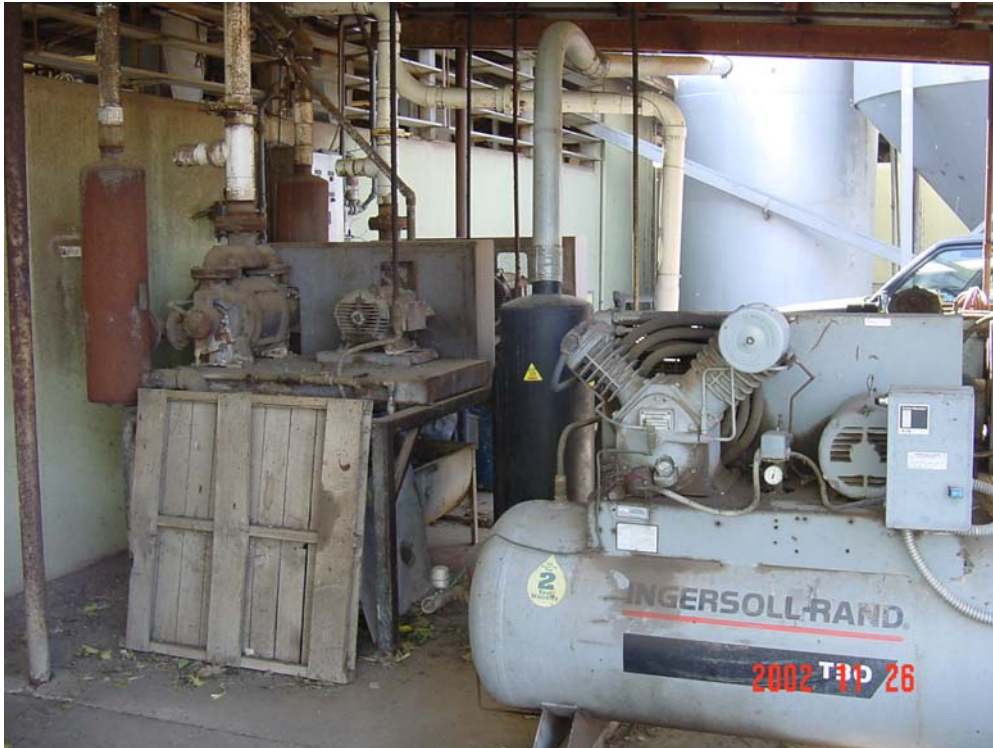
Overview Of Compressors.
