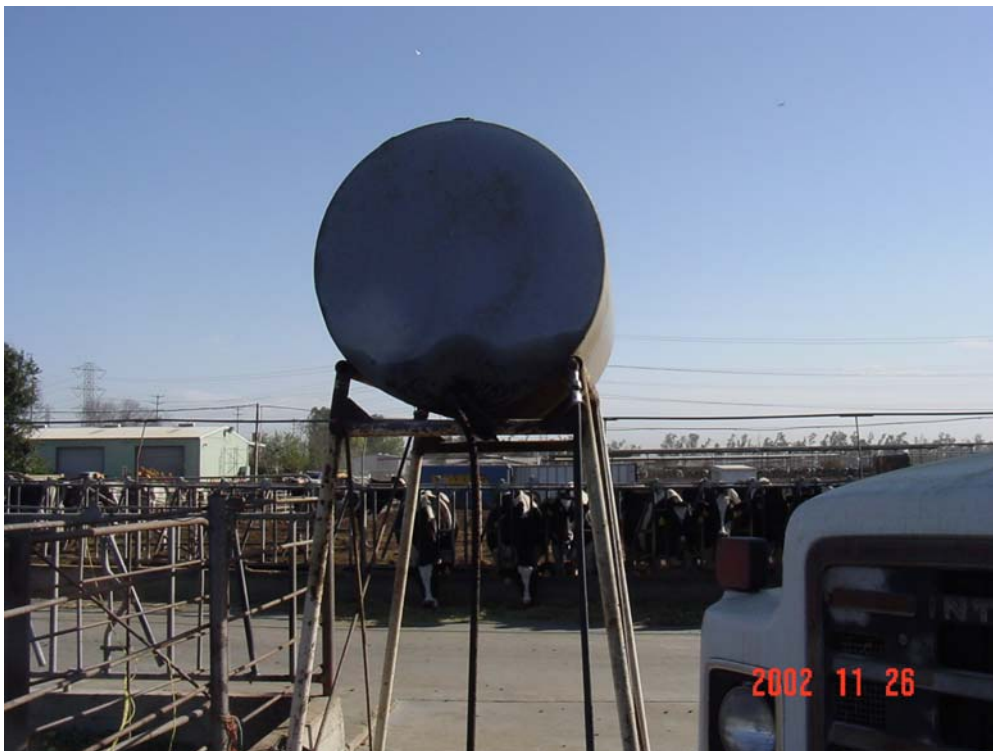
Overview Of Diesel AST.
