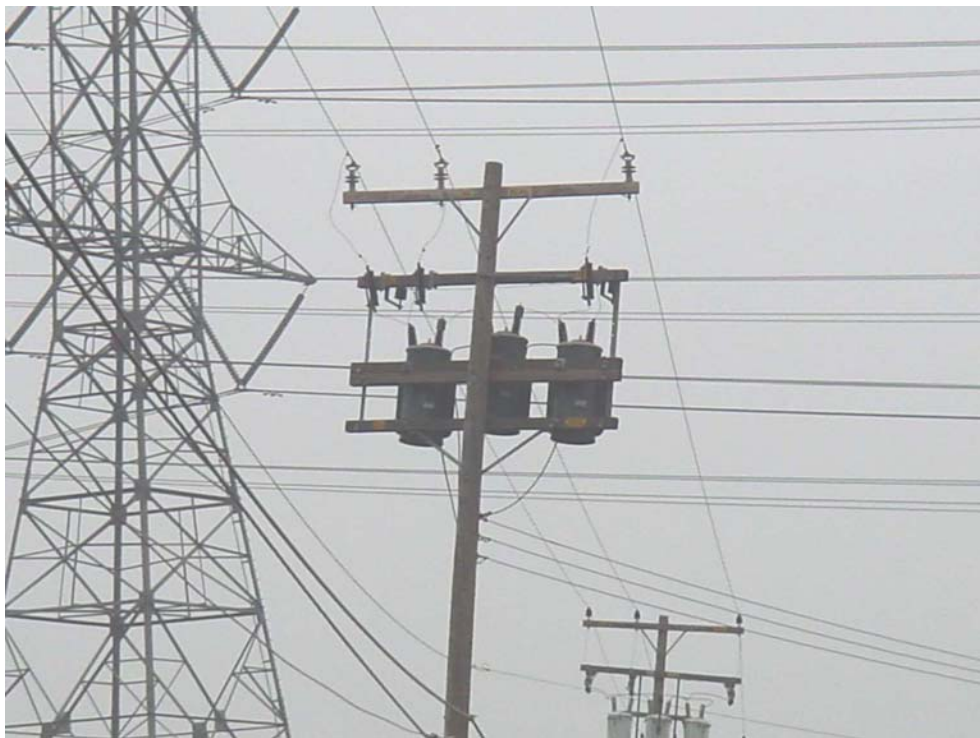
Close-up view of pole mounted transformers.
