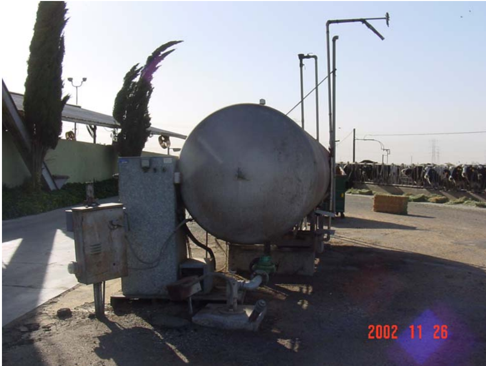
Overview Of Water Well And AST 1.
