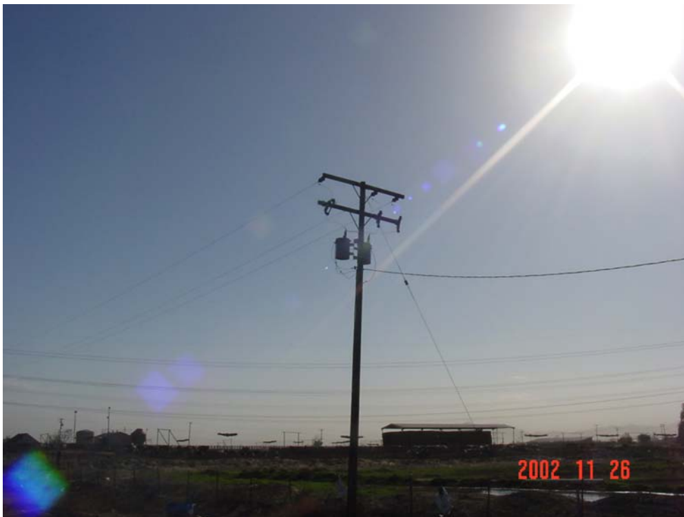
Overview Of Pole Mounted Transformers.
