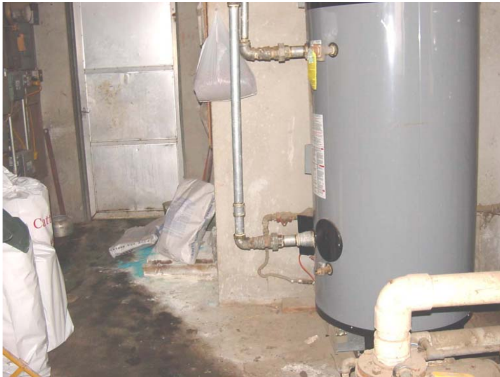
View of a water heater within the equipment room.
