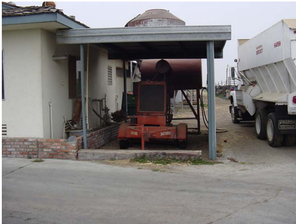
View of the emergency generator adjacent to the southeast corner of the milking barn.
