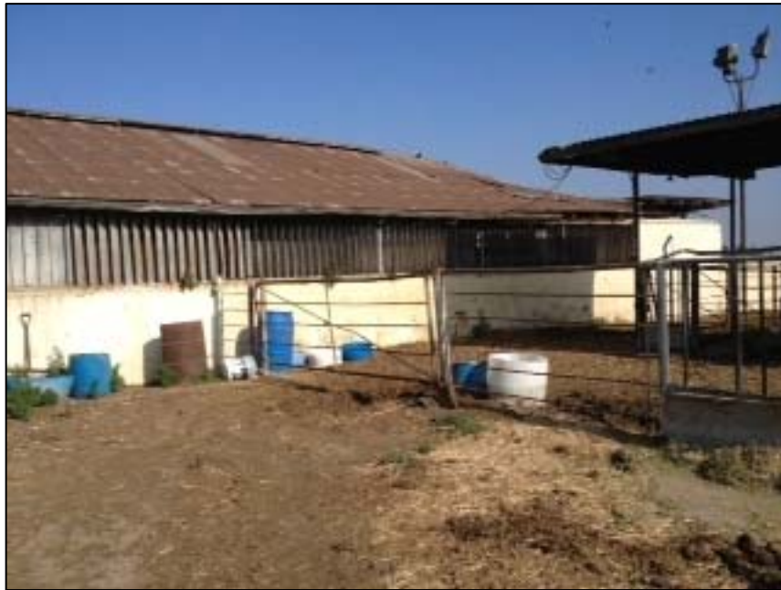
Photo taken of the northeastern side of Building B showing original stucco covered block walls, metal walls and corrugated iron roofing. All elements appear original.
