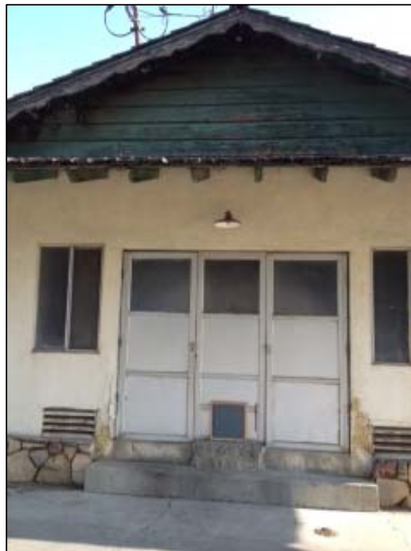
Close up view of the front of the Building B south façade. A two or three thousand gallon tank rests behind the door.
