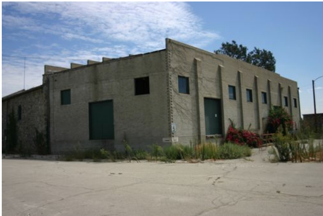
Building 54, north and west elevation, west end of building, view looking southeast, September 2008.
