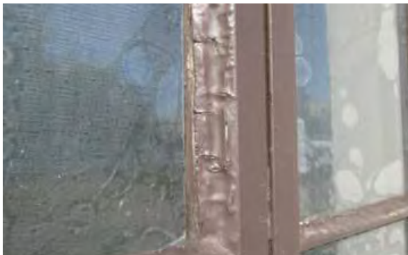
Typical condition at windows requiring basic maintenance; note cracked glazing putty.
