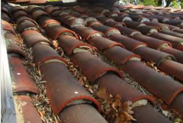
View of clay tile roofing from second floor window; note debris accumulation.
