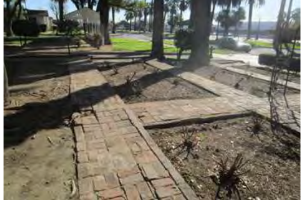
Damaged brick pavers at rose garden.
