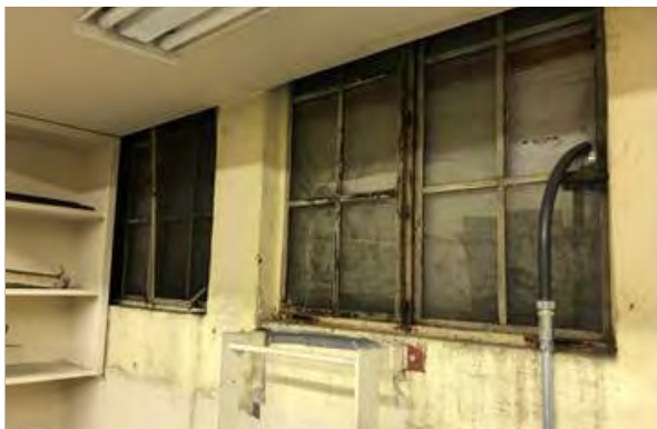
Deteriorated/damaged windows at basement. Windows covered with plywood at exterior.
