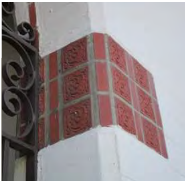
Typical terra cotta tile details flanking entrance bays at east courtyard elevation.
