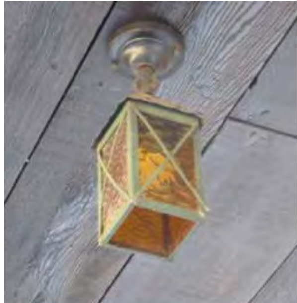
Typical bronze pendant fixture at courtyard veranda soffit.
