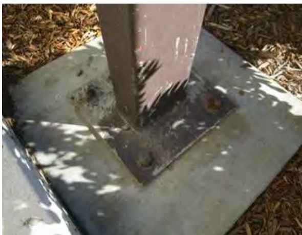
Base plate at steel column support; note corrosion at anchor bolts.
