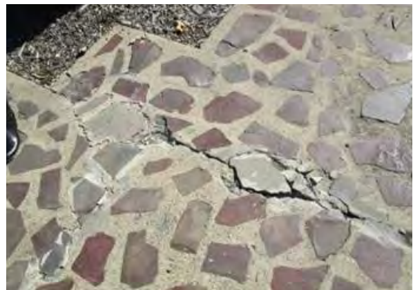
Cracking and spalling at slate paver walkway.
