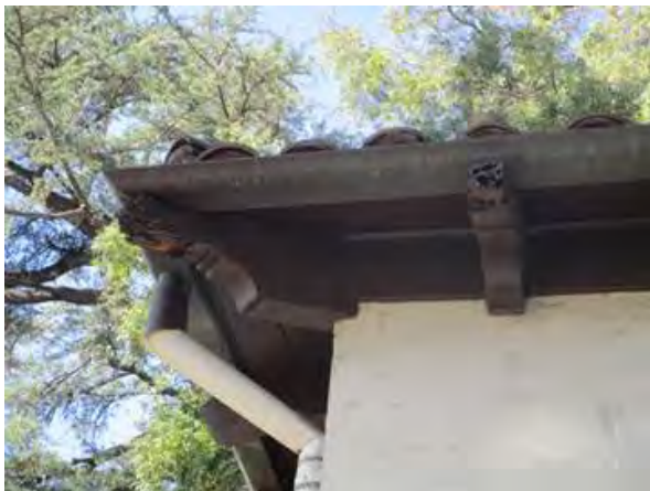
Typical decayed ends of exposed rafters. (northeast corner shown)
