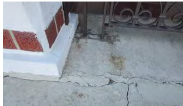
Detail view of damaged concrete.
