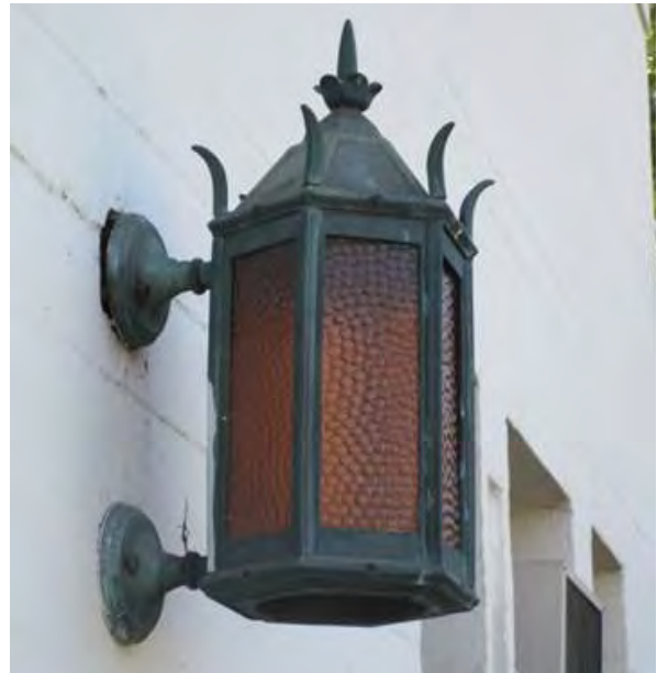
Bronze sconce at exterior entrance, east courtyard elevation; note missing lens at bottom, missing fasteners and localized corrosion products (green).
