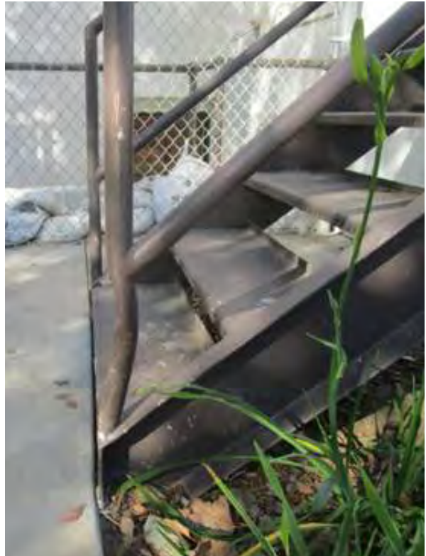
View of steel stair; note damaged rail post.
