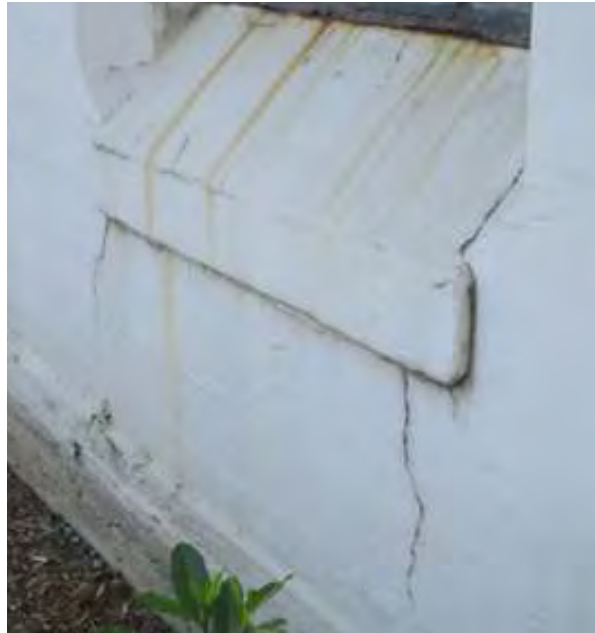
Cracks in concrete at west elevation.
