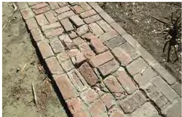
Uneven/deteriorated brick pavers and mortar joints.
