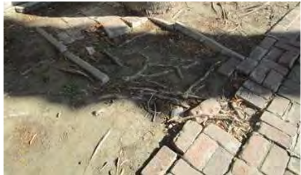
Walkway extension with missing brick pavers and tree root damage.
