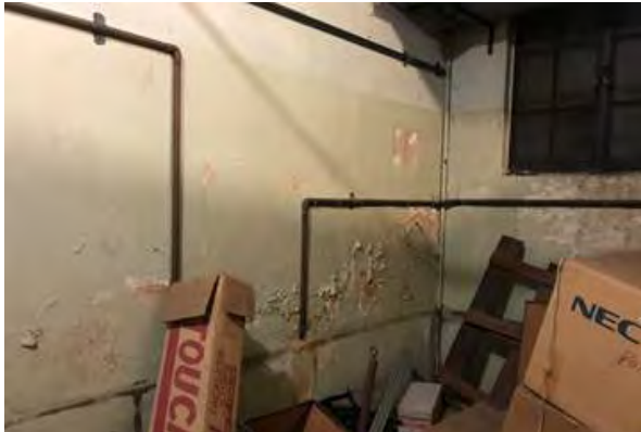
Peeling paint and deteriorated wall finishes at basement storage room.
