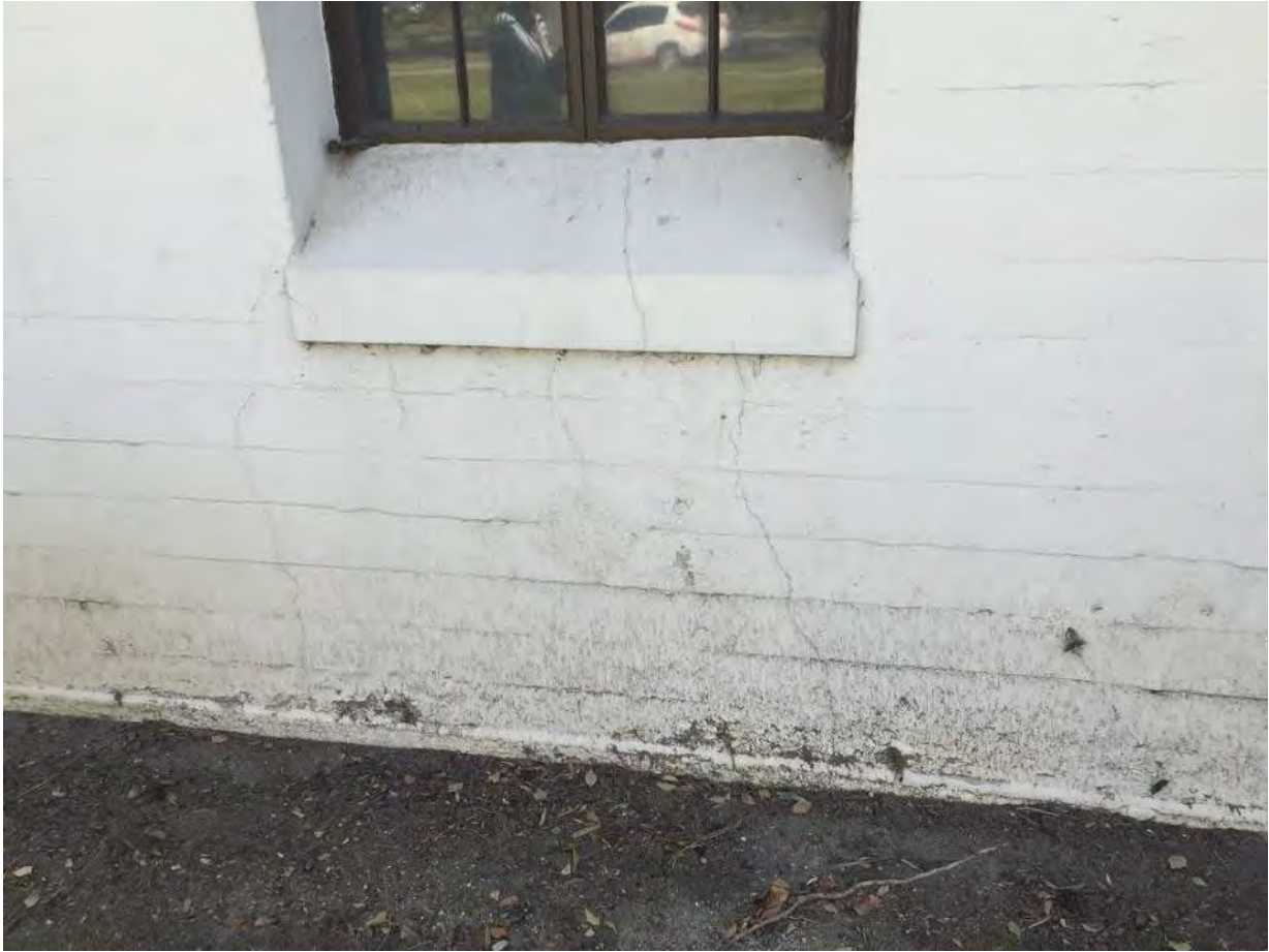
Image 6. Common crack pattern below exterior window.
