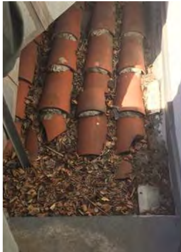
View from mechanical pad to clay tile roof at reported leak location. Note broken tile, heavy debris, and flashing.
