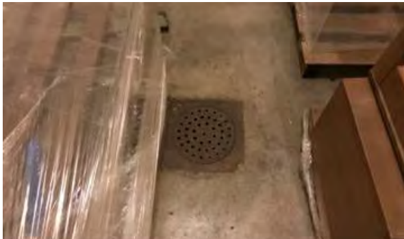
Typical floor drain at concrete floor slab in basement.
