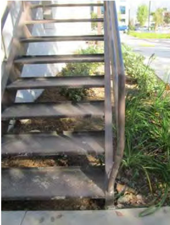
View of steel stair; note damaged rail post.
