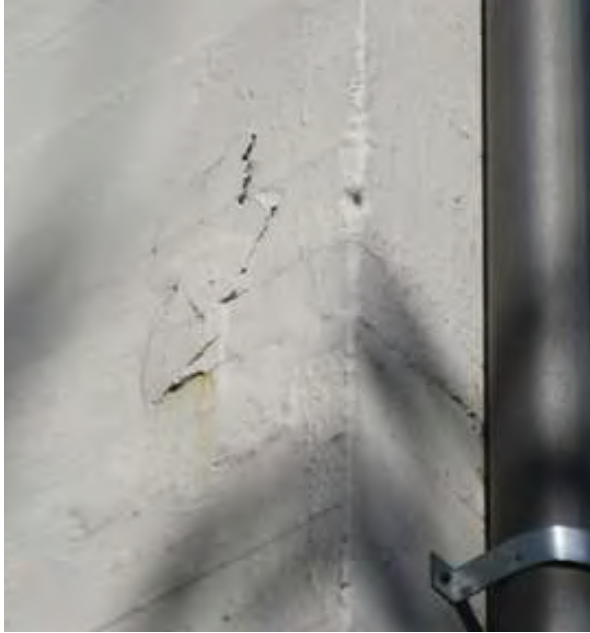
Spalled concrete at east elevation (south return).
