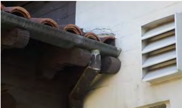
Gutter-to-downspout connection; note drip stains at loose fitting.
