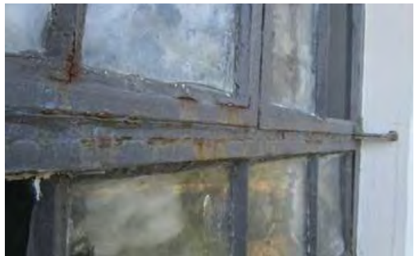
Typical condition at windows requiring more extensive repair; note corrosion of steel components.
