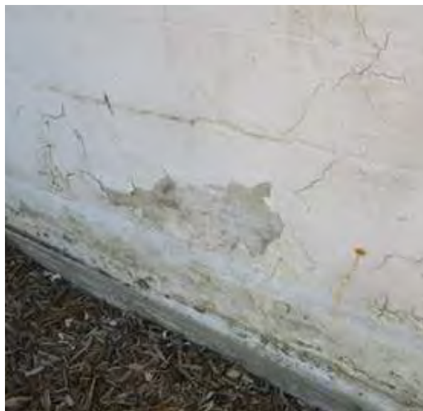
Peeled paint coating at base of wall, west elevation.
