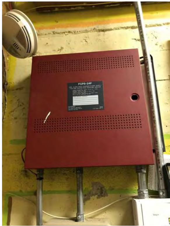
Figure 4 - Missing Fire Alarm Control Panel
