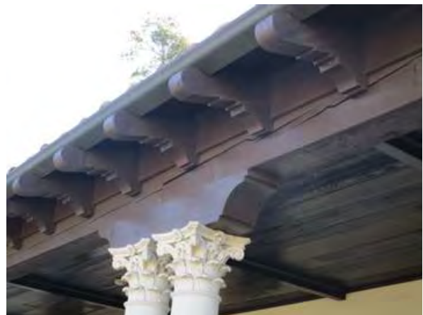
Typical deep checking/splits at veranda wood beams. (south courtyard elevation shown)
