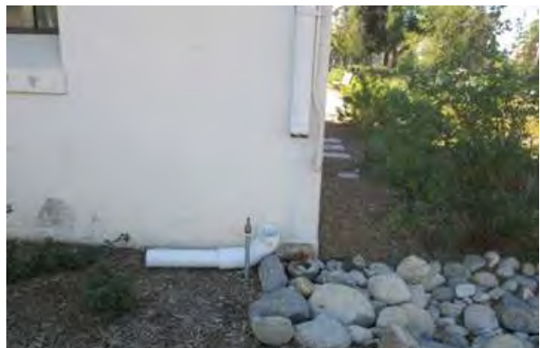
Replacement PVC extension disconnected from downspout at northwest corner of building.
