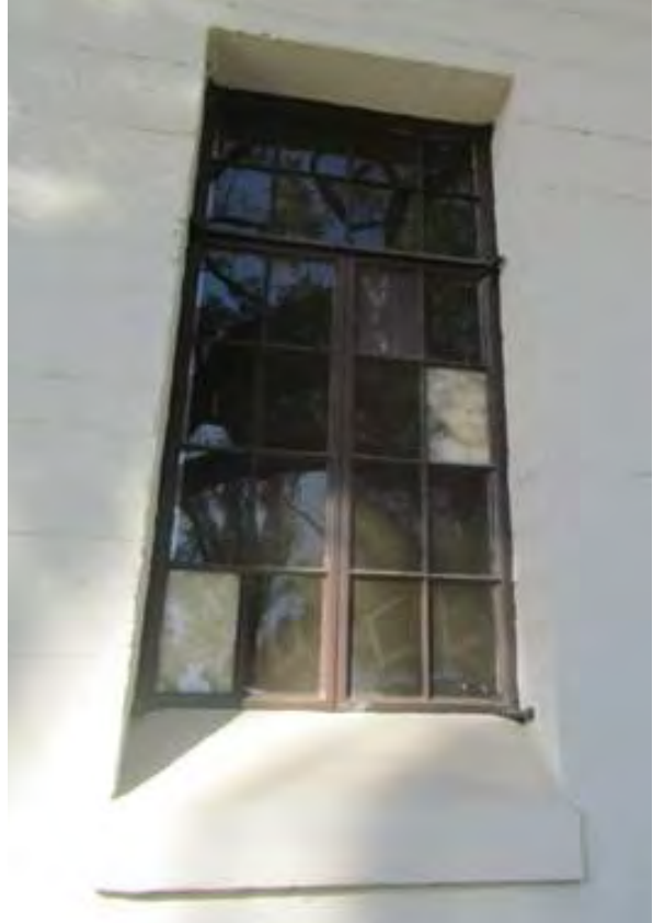
Typical window at gallery blocked with interior partition; note insulation fill and back-painted glass.
