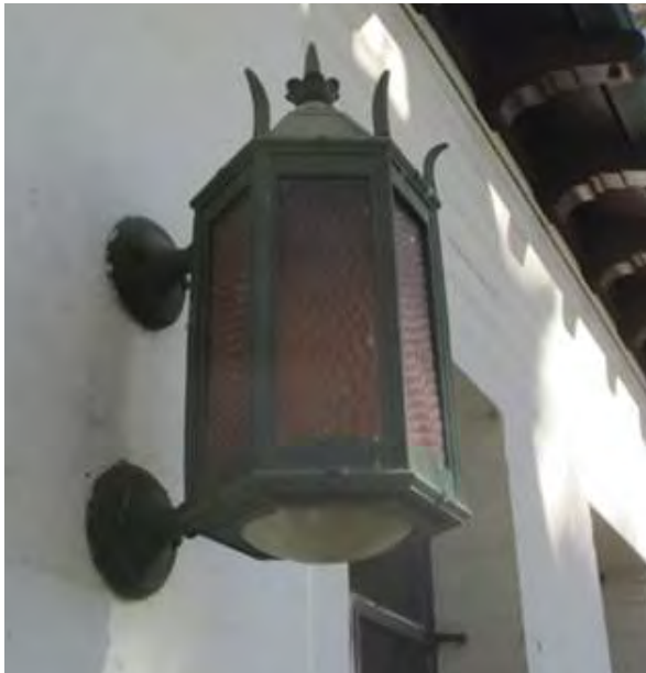
Bronze sconce at exterior entrance, south elevation; note heavy soiling.
