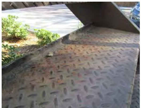
Checker-plate steel stair tread; note surface corrosion and peeling paint.
