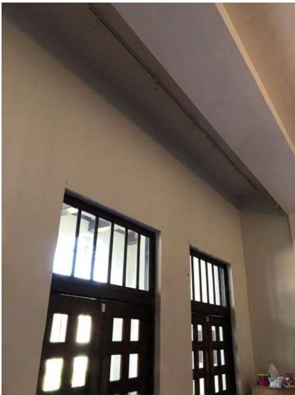
Figure 3 - Sample Missing Exit Sign/Emergency Fixture
