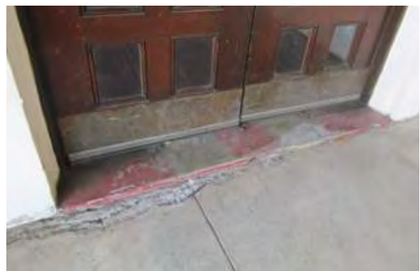
Typical concrete spalling at entrance thresholds, north and south courtyard elevations.
