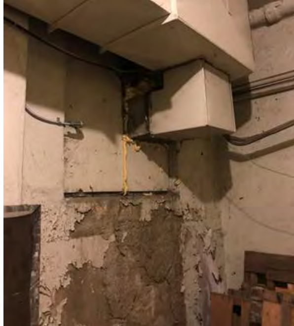
Ductwork installed in basement window opening. Note plywood infill, sealant, and heavy deterioration of wall below.
