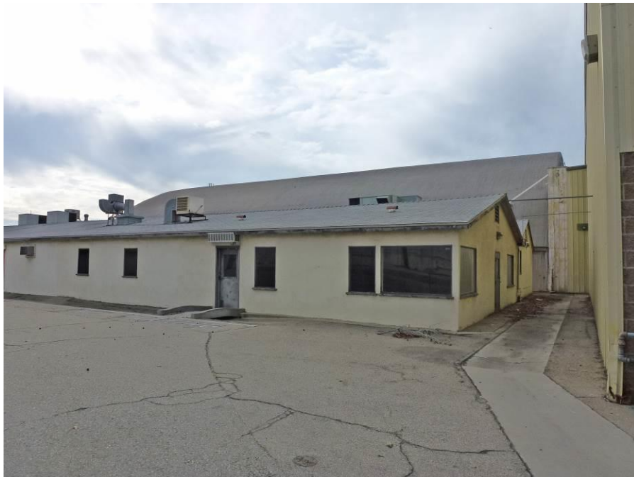
Image 2. View looking south at the northwest and northeast facades of the Commissary Building, with Hangar 3 in the background. ASM, December 1, 2016.
