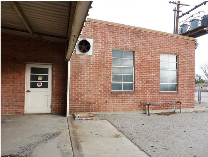
Image 7. Detail view looking east at the west façade of the Diesel Tanks room.
