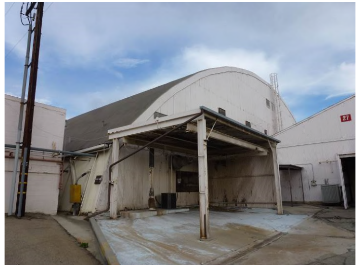
Image 4. View looking north at the southwest and southeast façades of Hangar 3 and the steam clean shed.
