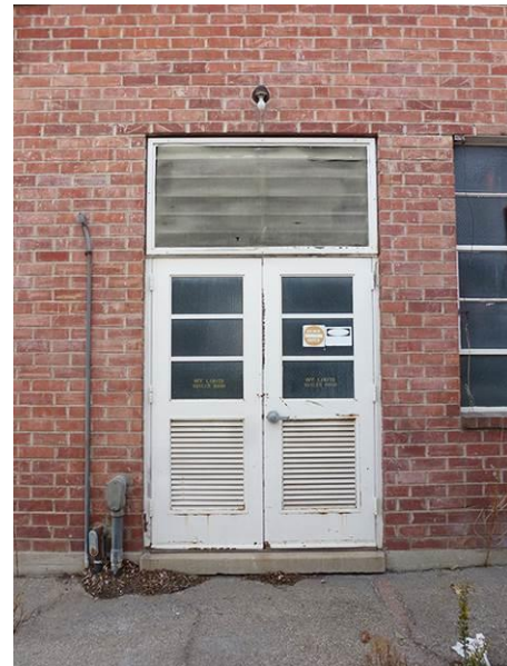
Image 8. Detail view of the entrance on the east façade of the Diesel Tanks room.
