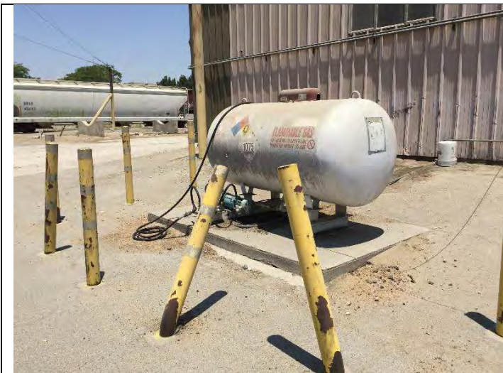
11. View of Propane near Warehouse Building (Building C)
