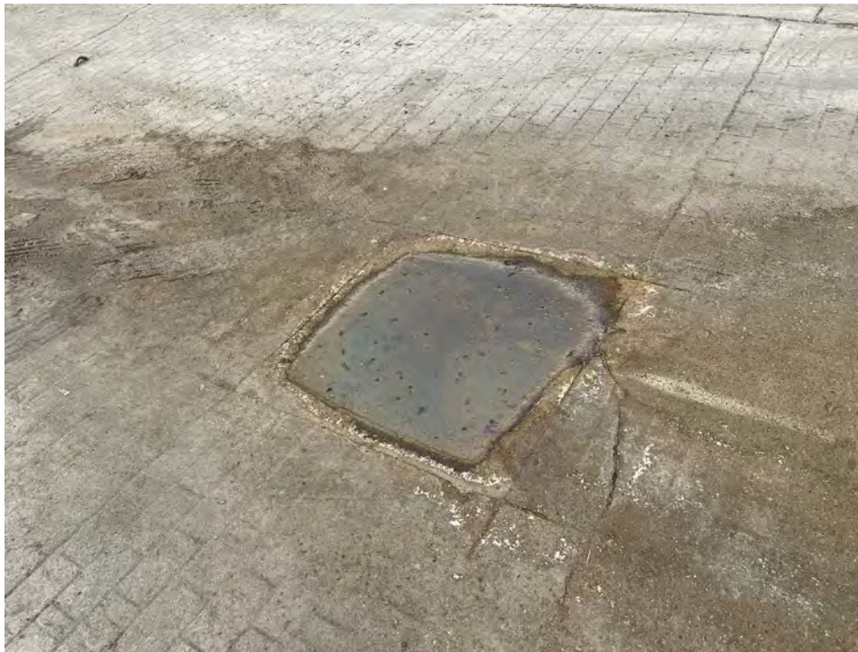
Photograph 4: Sump in truck-washing area.
