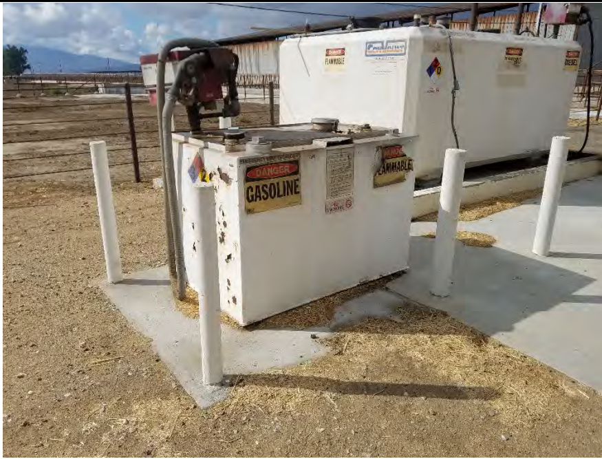
15. Additional photo of 2,000-gallon AST and 240-gallon AST.
