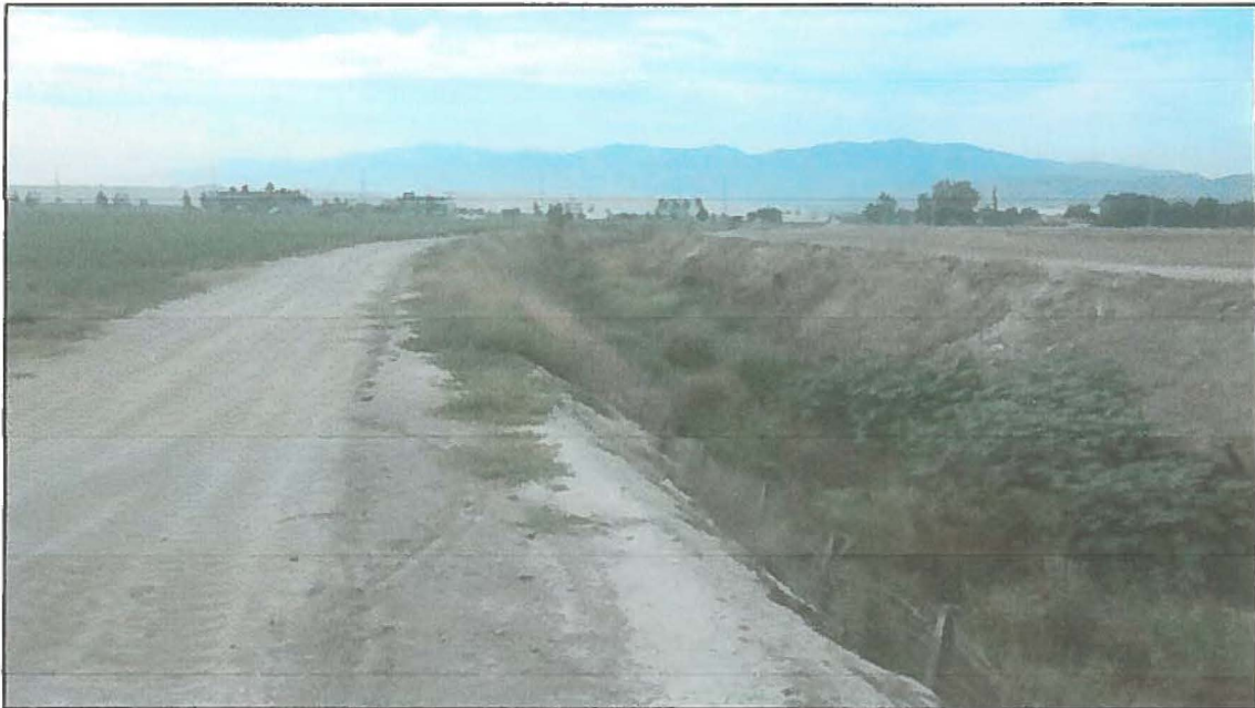
View south of the Cypress Channel north of Kimball showing the cut walls, railroad tie shoring and wire fence.
