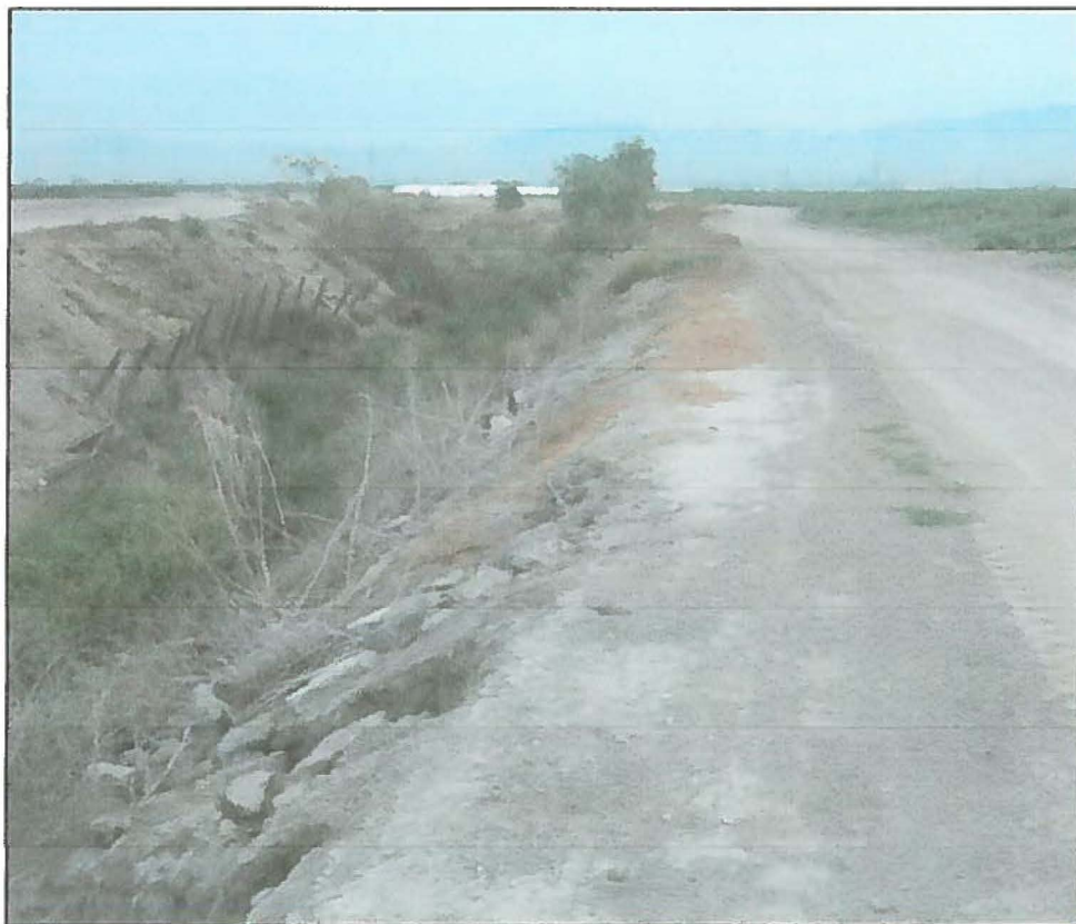
View north-northwest of the Cypress Channel showing the cut walls, railroad tie shoring and wire fence.
