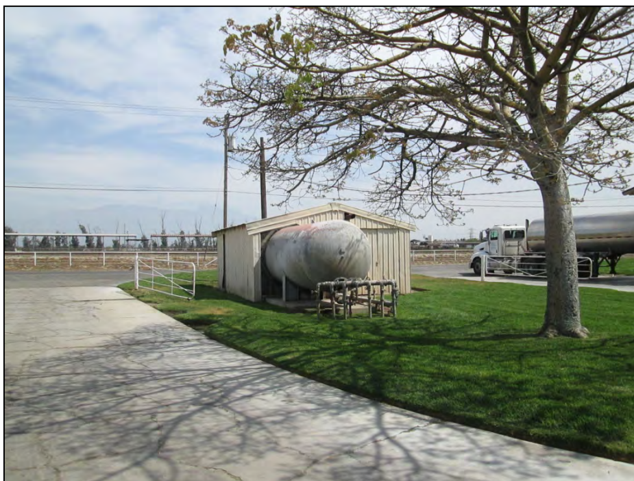
Water pump and tank located immediately west of Auxiliary Dairy Barn. View looking north
