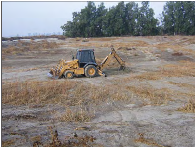
Southwest Wastewater Pond
