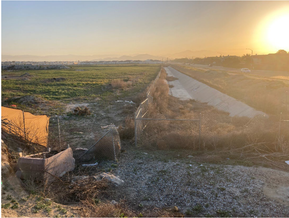
Photo 11: View of flood control channel located south of the Project Footprint, east of Haven Avenue; facing east. March 2022.
