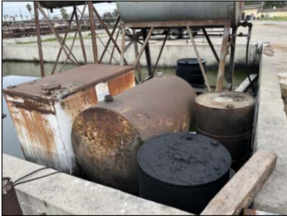
View of ASTs and 55-gallon drums in hazardous materials storage area.
