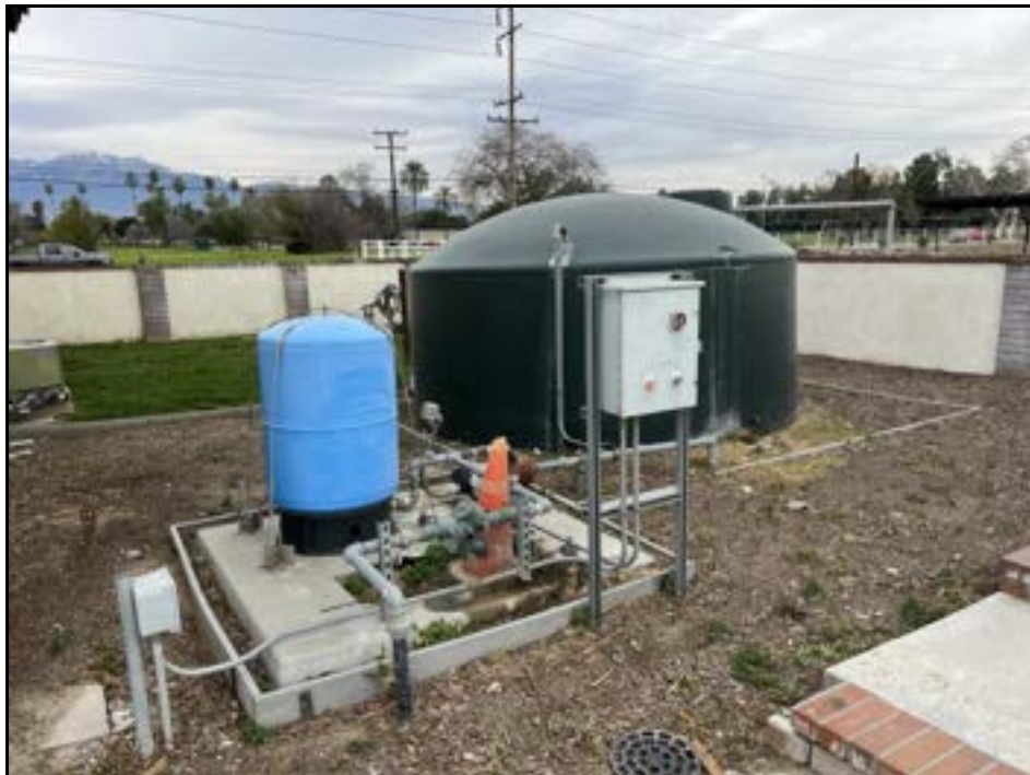
View of drinking water holding tank adjacent to main residence in northern portion of Subject Property.
