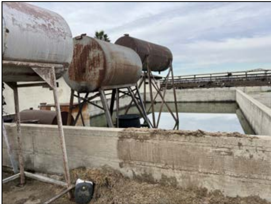
View of concrete-bermed hazardous materials storage area with standing water from recent rains.
