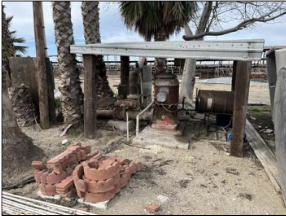
View of private well in northeastern portion of Subject Property.
