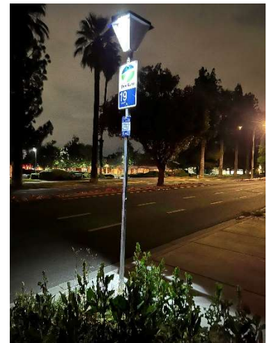
Figure 6-10 - a standard solar light in Omnitrans' service area.
