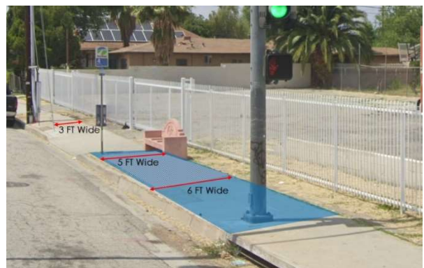
The landing pad does not adhere to ADA standards. Additionally, the bench partly obstructs it. The path of travel is narrow and cramped, and the sidewalk is not very accommodating.
