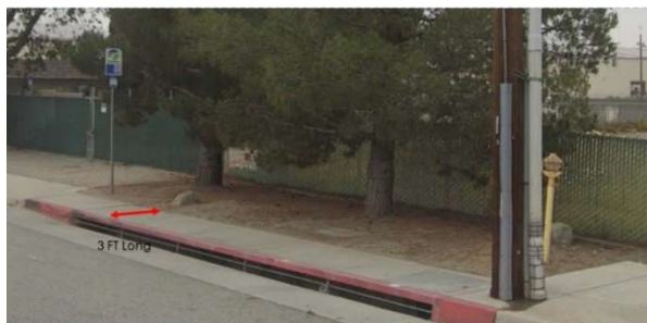
Landing pad is less than 3 ft wide.
