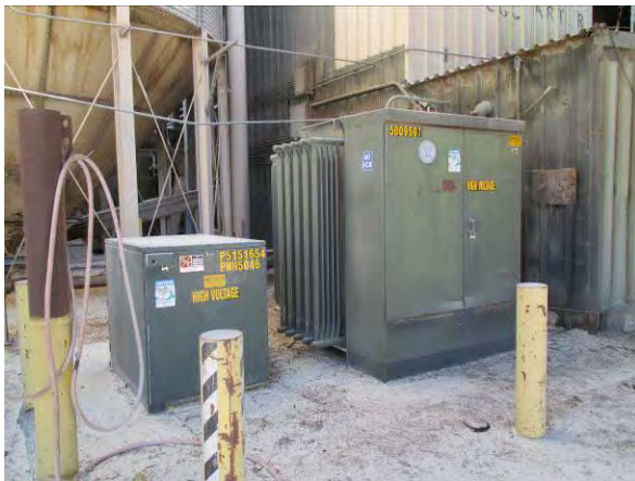
Photo #21 View of the pad-mounted transformer.
