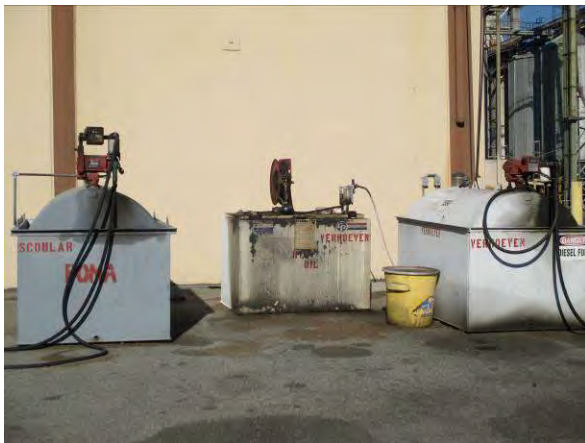
Photo #15 View of three ASTs located on the exterior eastern side of the office/warehouse building.
