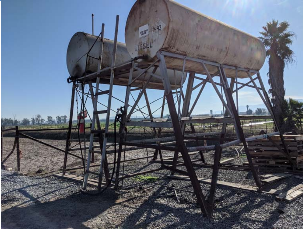
PHOTO 9: View of the elevated ASTs at the Site.
