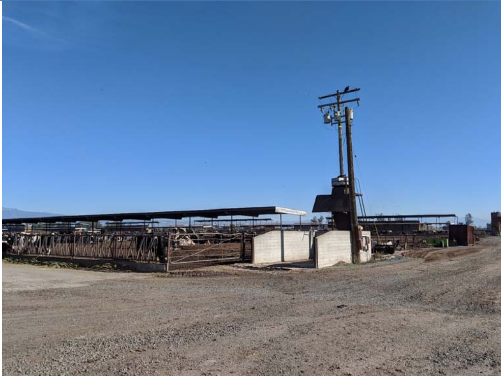
PHOTO 11: View of the corrals and the pole-mounted transformers at the Site.
