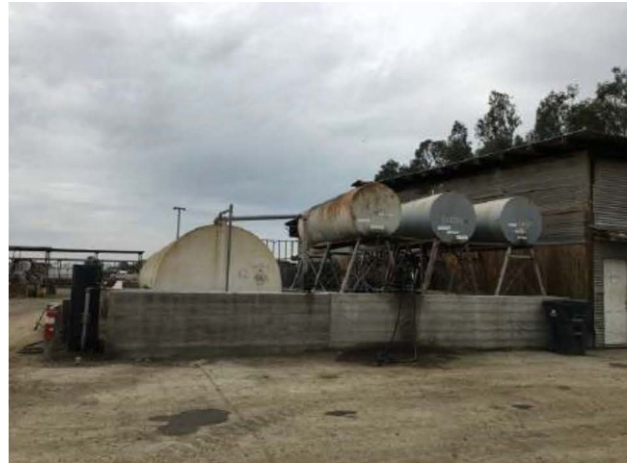
View of 10,000-gallon and three 1,000-gallon diesel ASTs for fueling.
