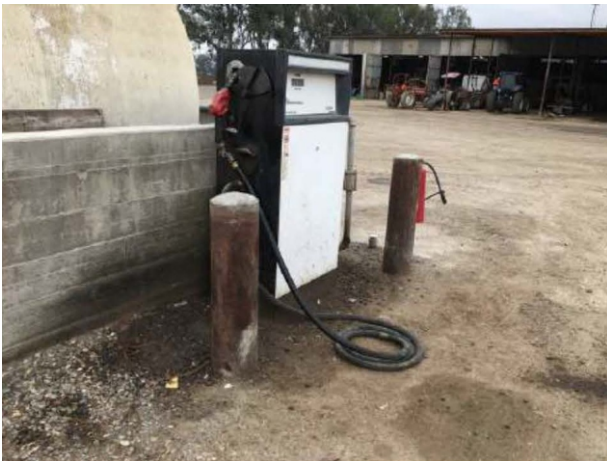
View of fuel pump for the 10,000-gallon diesel AST with staining around the base.
