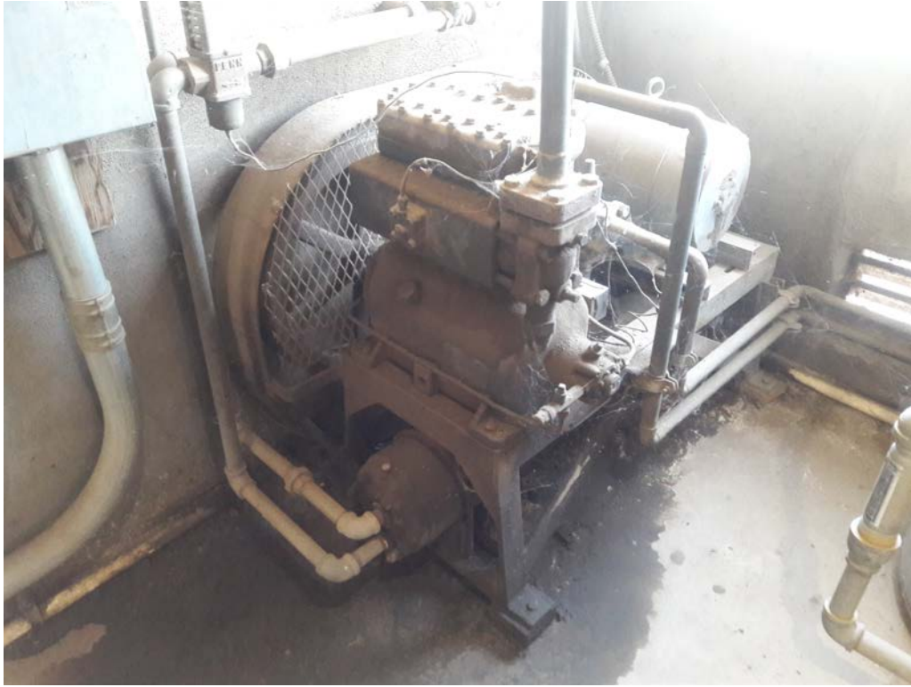
Photo #21: View of the generator and associated oily staining located in the northeastern milk barn.
