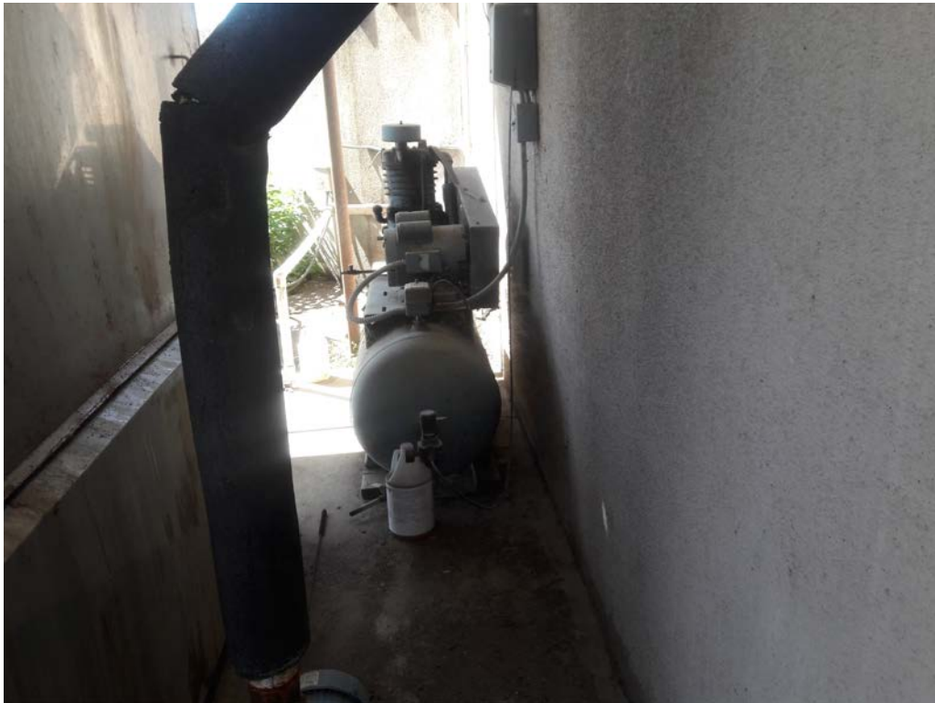
Photo #22: View of the air compressor located outside of the northeastern milk barn.
