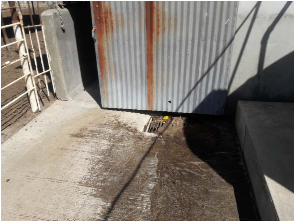
Photo #25: View of the clogged drain located on the southern side of the western milk barn.
