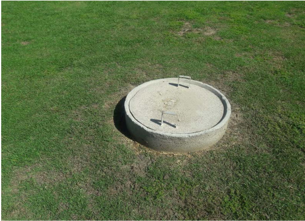
Photo #5: View of the unknown manhole located north of the northeastern milk barn.
