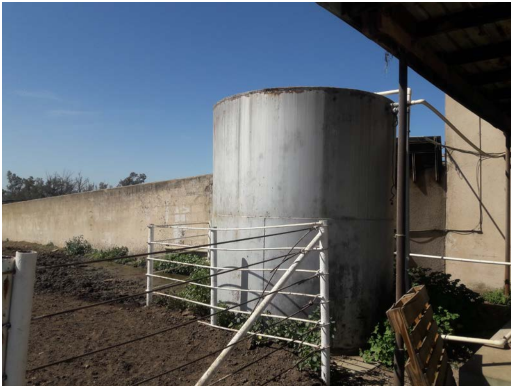
Photo #20: View of the water AST located on the southeastern exterior of the northeastern milk barn.
