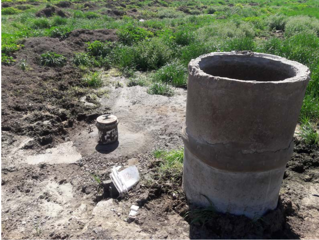
Photo #19: View of the unknown cleanout and manhole with standing water located in the southern portion of the Subject Property.
