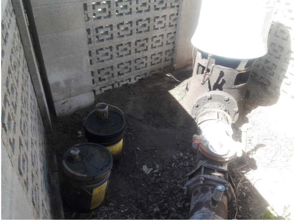
Photo #3: View of the well that supplies potable water to the residential structure with storage of chemicals and associated staining.
