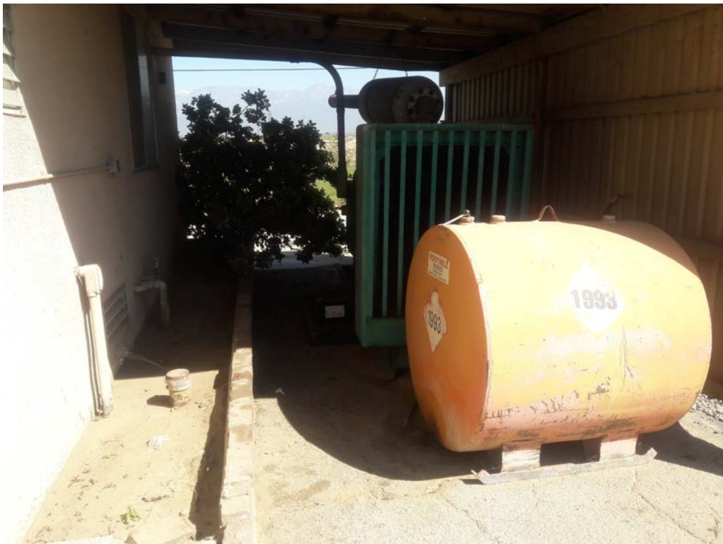
Photo #6: View of the backup generator and associated approximately 500-gallon diesel AST located on the eastern side of the northeastern milk barn.
