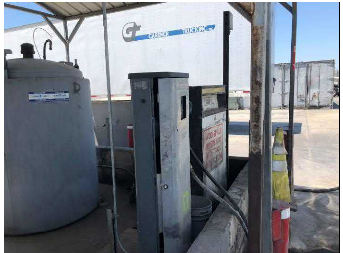
40. View of fuel dispenser.
