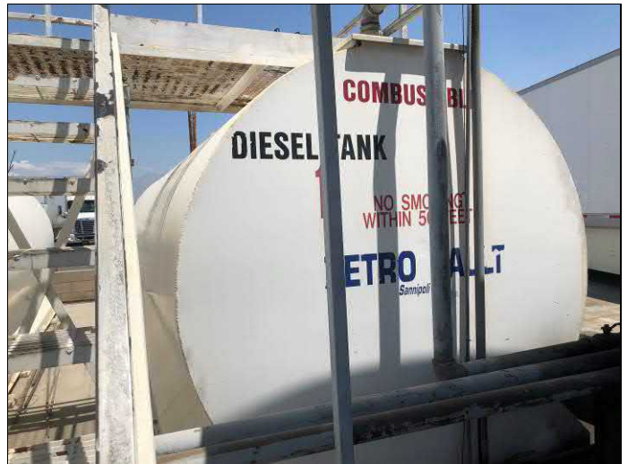
34. View of 8,000-gallon diesel AST in fueling area.
