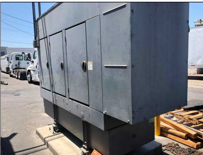
17. View of diesel-powered generator by service area and office.
