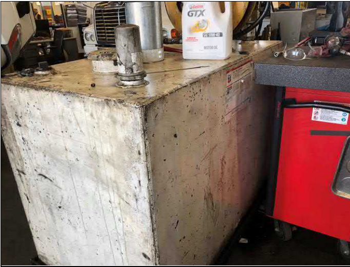
7. View of approx. 500-gallon new antifreeze AST.
