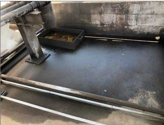
39. View of petroleum staining in bermed area.
