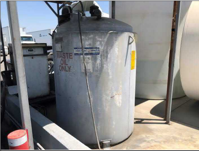
37. View of waste oil AST in fueling area.
