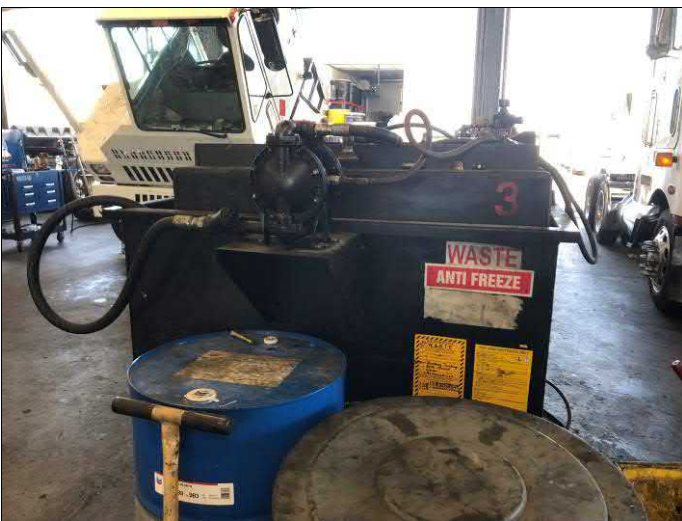
5. View of approx. 500-gallon waste antifreeze AST.
