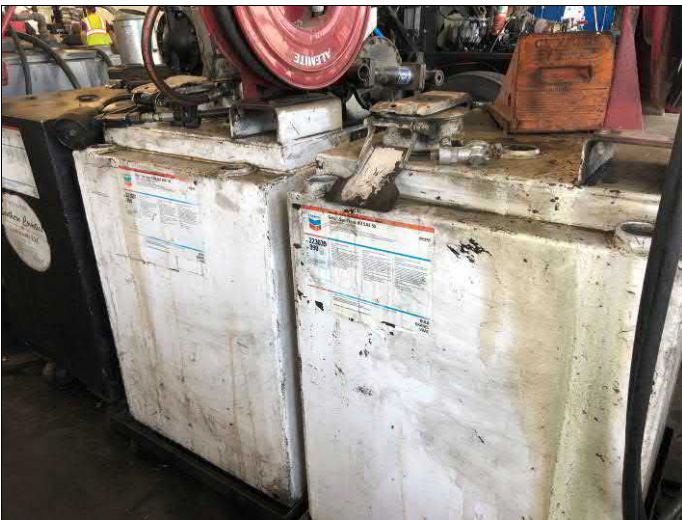
3. View of approx. 75-gallon double-walled ASTs containing gear oil (x2) and transmission fluid (x1).
