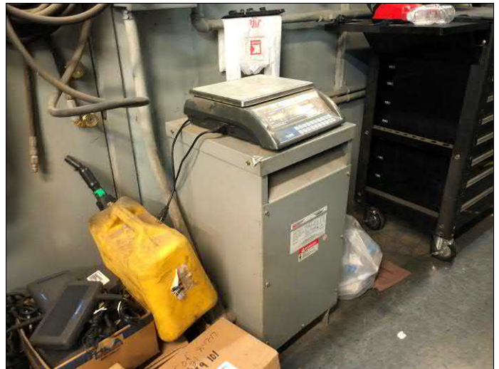
16. View of transformer in office.
