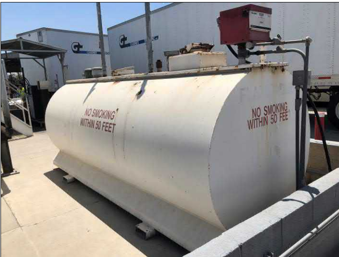
33. View of 6,000-gallon diesel AST in fueling area.
