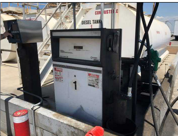
41. View of additional fuel dispenser.
