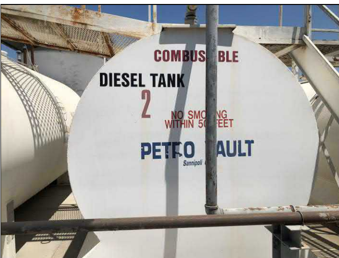
35. View of 8,000-gallon diesel AST in fueling area.
