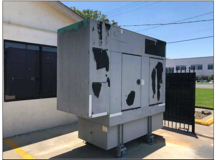
20. View of diesel-powered generator by administrative building.
