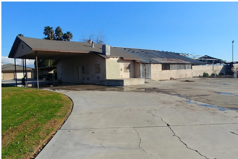
Plate 3.2-32: Overview of the Site Temp-15 milk barn at 14651 Grove Avenue, facing northeast.
