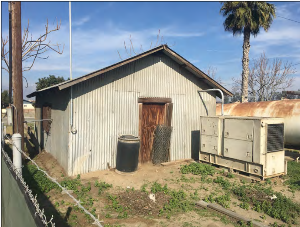
View northeast of ancillary shed, south and west facades, January 2020. Source: Urbana Preservation & Planning, LLC.
