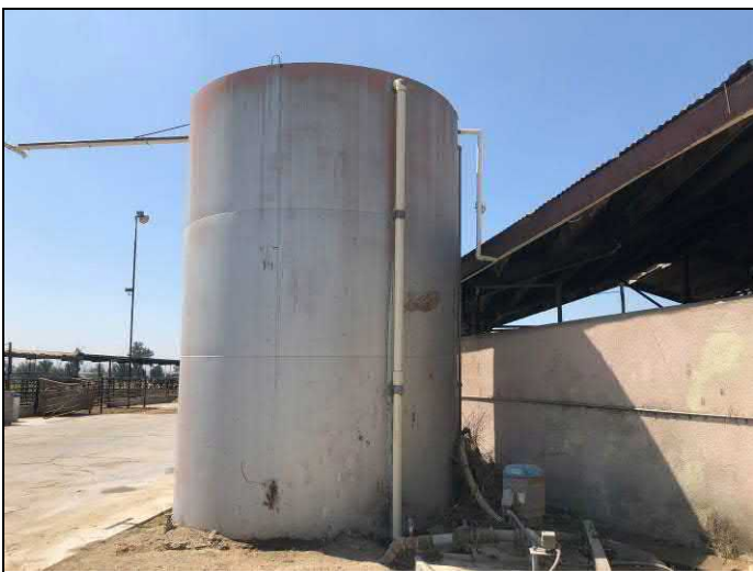
11. View of new washwater storage tank.
