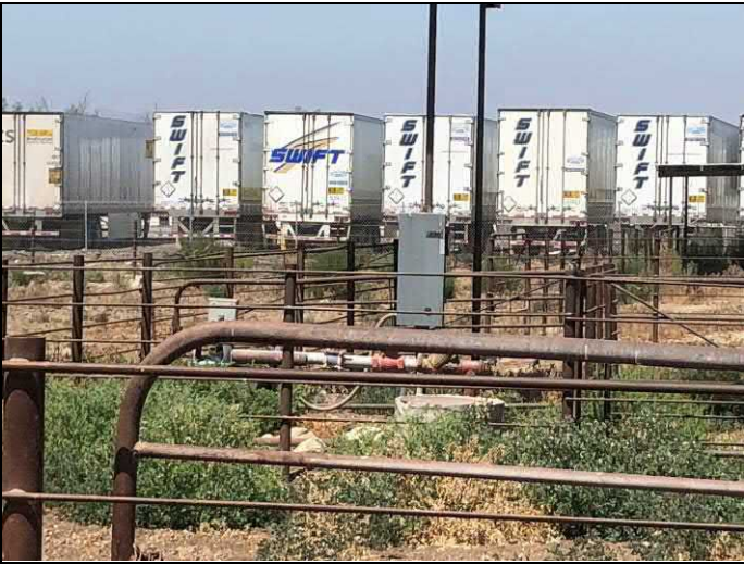
19. View of electrical irrigation/domestic well.
