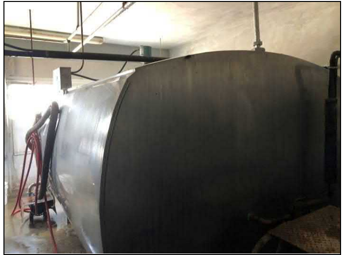
8. View of additional milk storage tank.
