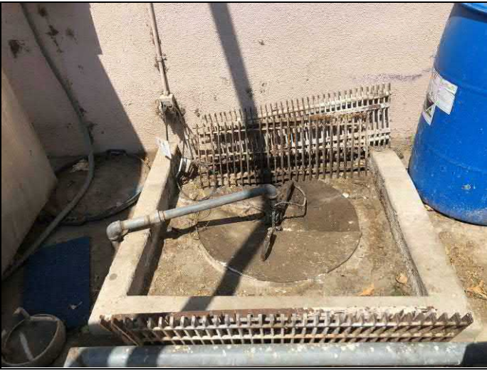
13. View of sump for runoff from cooling system.
