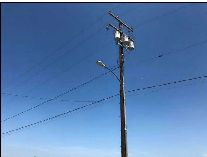
23. View of pole-mounted transformers.
