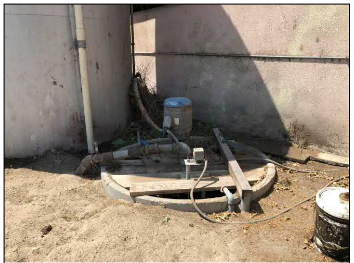
12. View of washwater pump.
