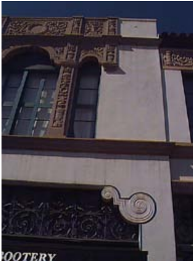
Highly detailed facade ornamentation adds to the building character. Note the detailing on the transom window is derived from the facade ornaments.
