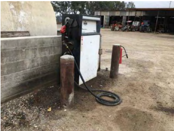
View of fuel pump for the 10,000-gallon diesel AST with staining around the base.
