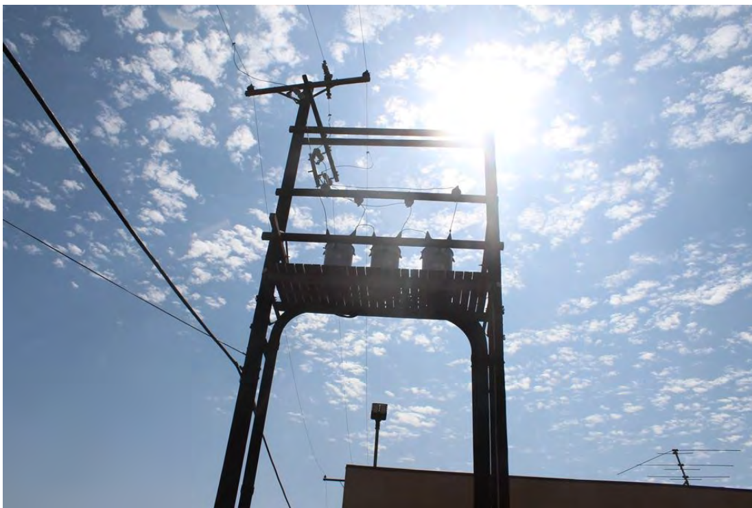
Overview of power poles at center of site.
