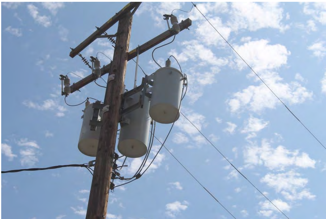
Overview of power pole at center of site.
