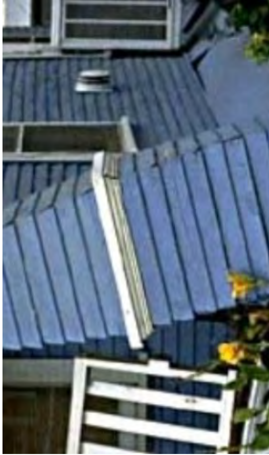
Figure 4-16: Earthquakes can be so strong they knock houses and buildings off their foundation.
