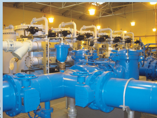
John Galvin Ion Exchange Treatment Plant
