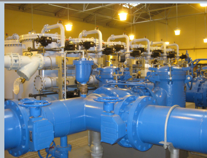
John Galvin Ion Exchange Treatment Plant Placed into Service in October 2009
