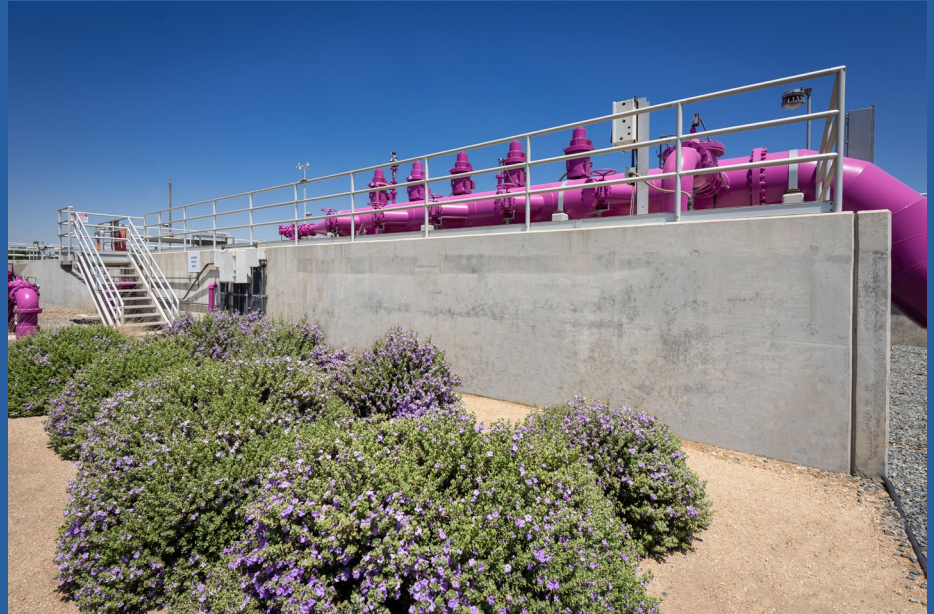
Steel Recycled Water Pipes, n.d. Digital print Courtesy of the Inland Empire Utilities Agency
