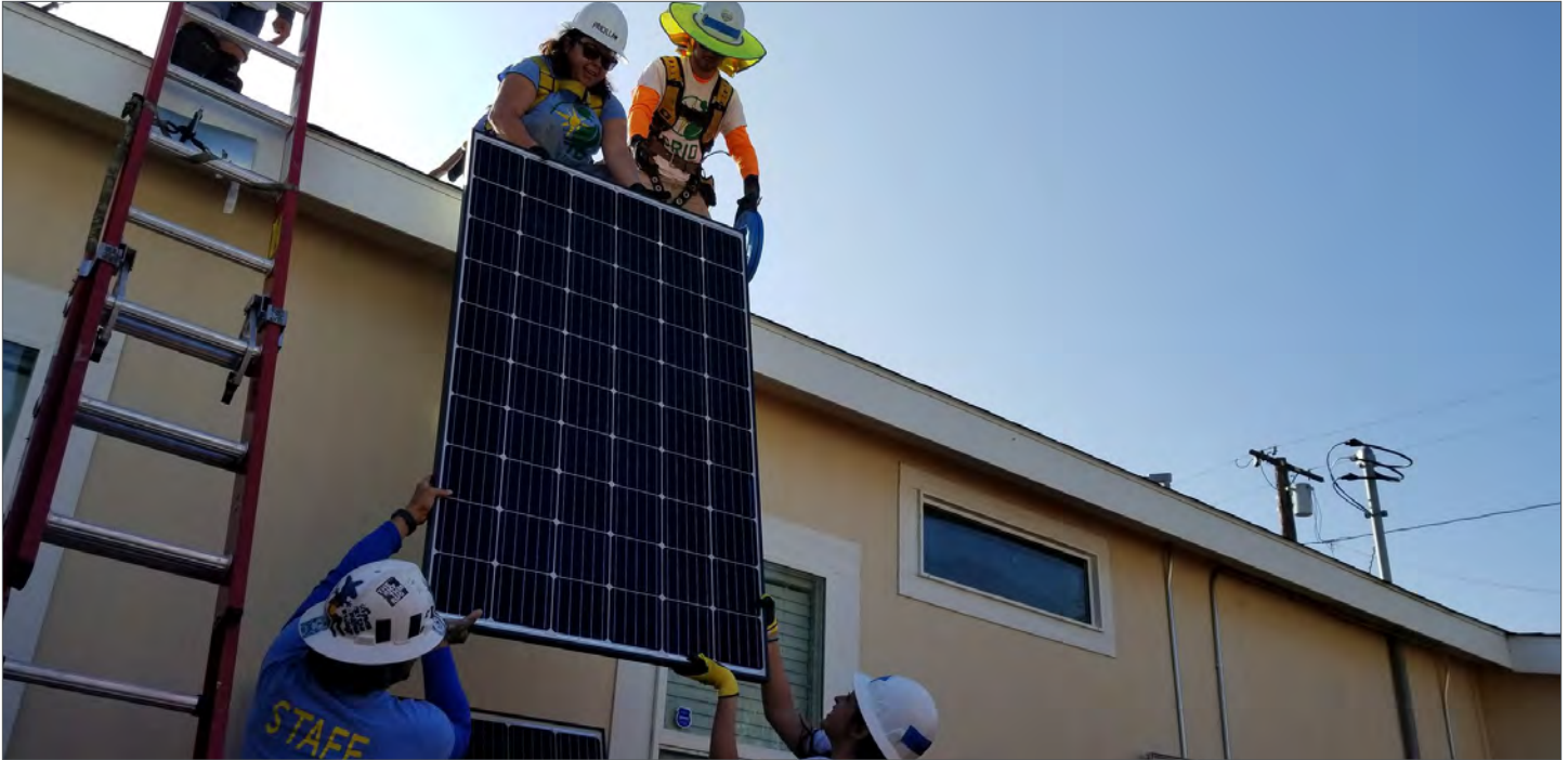
GRID Alternatives staff and trainees install rooftop solar PV panels in July 2019. Photo credit: GRID Alternatives
