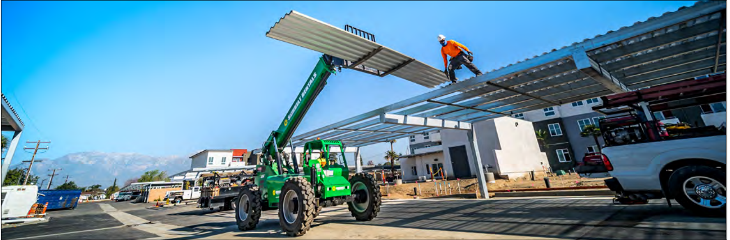
Construction of shade structures at Vista Verde Apartments in January 2021, which will also support an array of solar panels.
